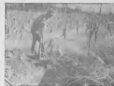
When a break is reported by the flying inspector, a repair crew gets on the job. Here a crew man uncovers sections of pipe at the site of the break, and prepares to restore the line.
